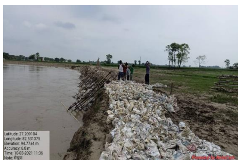
Mitigation of flood through a Bamboo grids + sandbag check dam at Sekhuia village
