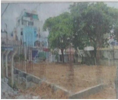
Encroachment of lake for building construction
